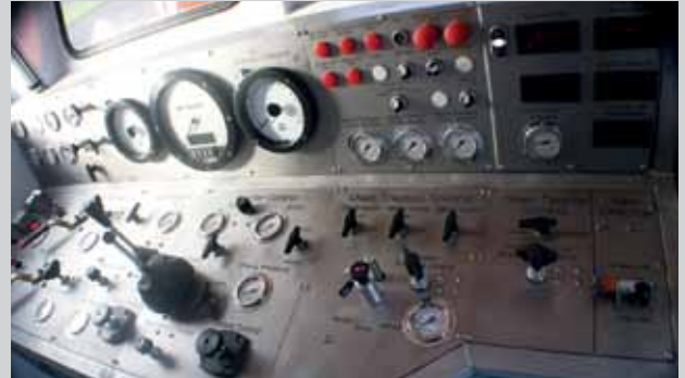
CTU Control Panel
