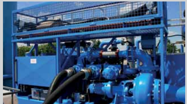
Discharge Side View
